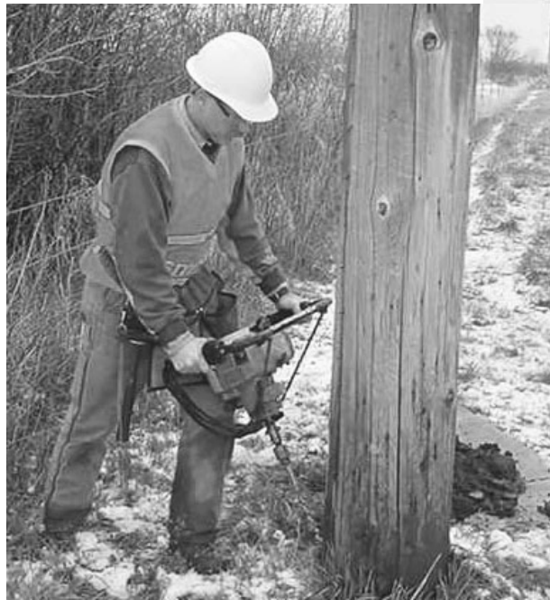
Pole inspection crews inspect utility poles to ensure poles are in good condition.
